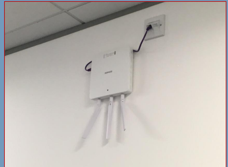
Wall mounted office Wi-Fi Access Point
